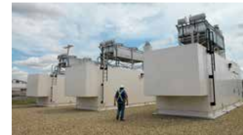
9 Landfill Gas Recovery System Captures and converts landfill gas into electricity – enough to power up to 4,600 homes annually.
