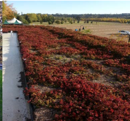
Valley Zoo Entry Plaza Green Roof in Edmonton, AB. Photo by Kenneth Yip, City of Edmonton 2014
