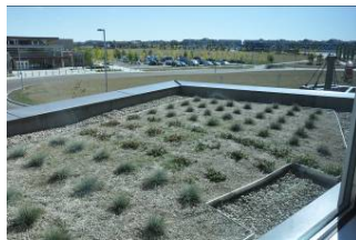
Newly planted green roof at Terwillegar Recreation Centre showing perimeter drainage, Edmonton, AB. Photo by Xiangfei Li, City of Edmonton, 2011.
