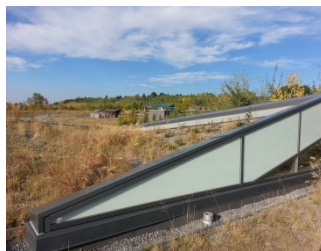
Green roof at Valley Zoo Arctic Shores in Edmonton, AB. Photo by Kenneth Yip, City of Edmonton, 2014.
