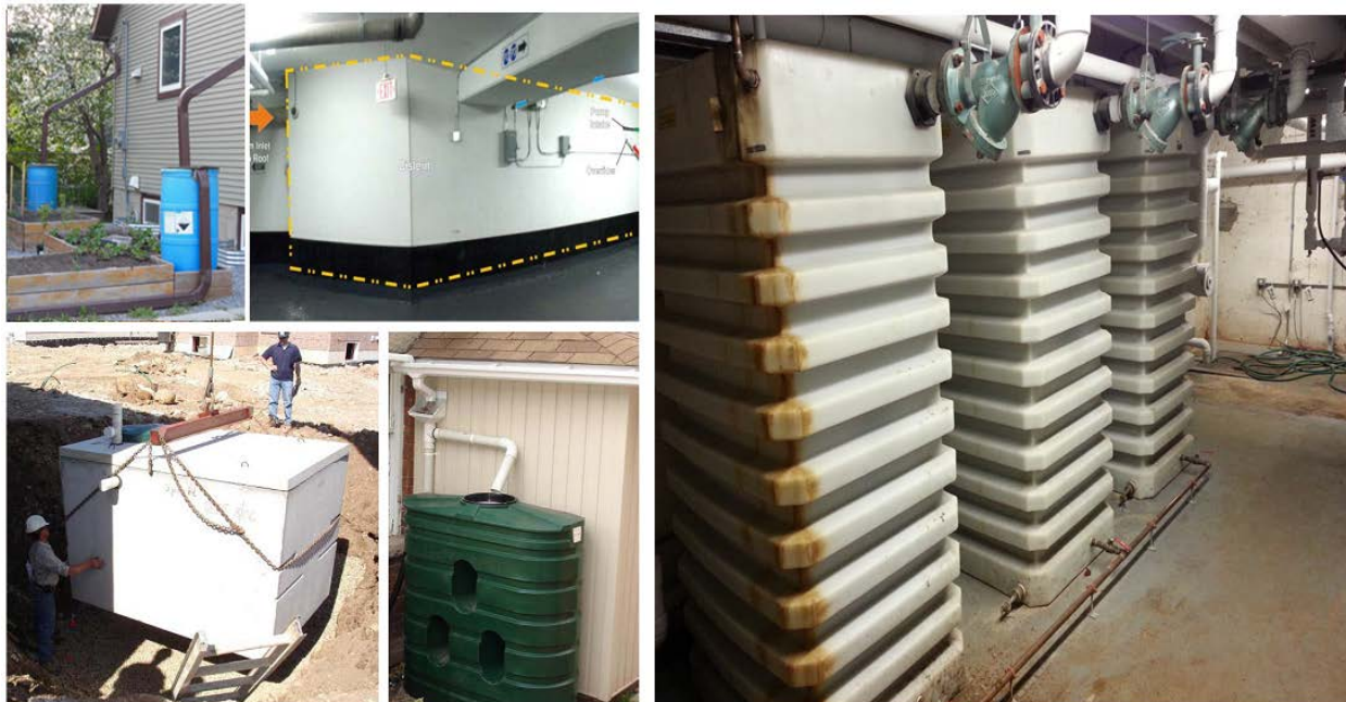
Clockwise from top left: Residential rain barrels, photo by Diane Wirtz, 2013; cast in place concrete cistern integrated within a parking garage (Source: TRCA); above-ground plastic cistern; underground pre-cast concrete cistern (Source: University of Guelph)
