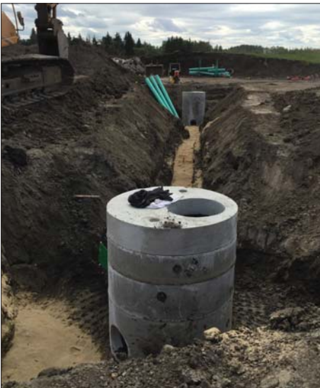
An example of utilities excavation that may be required for this project.
