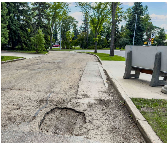
Asphalt failure along 142 Street service road
