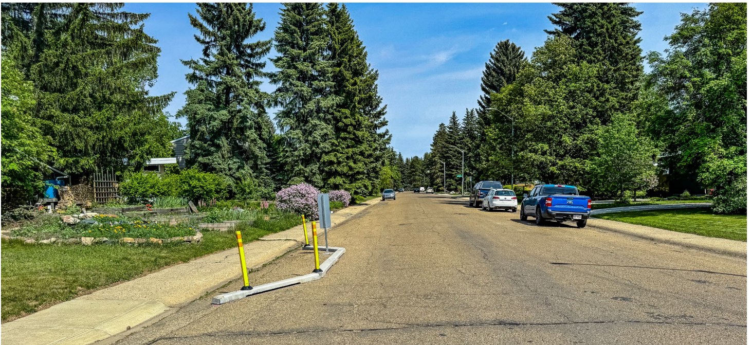
Temporary curb extensions on 89A Avenue were part of the Street Lab and will be reviewed during Neighbourhood Renewal
