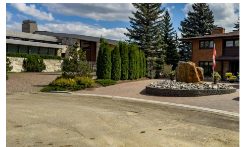
Missing sidewalks on Valleyview Point
