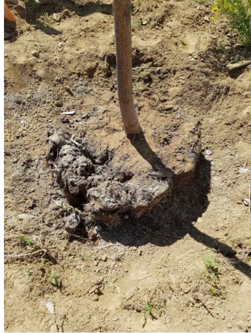
Improper Tree Planting
