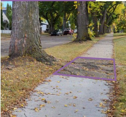
Figure 4 Sidewalk buckling caused by tree root encroachment
