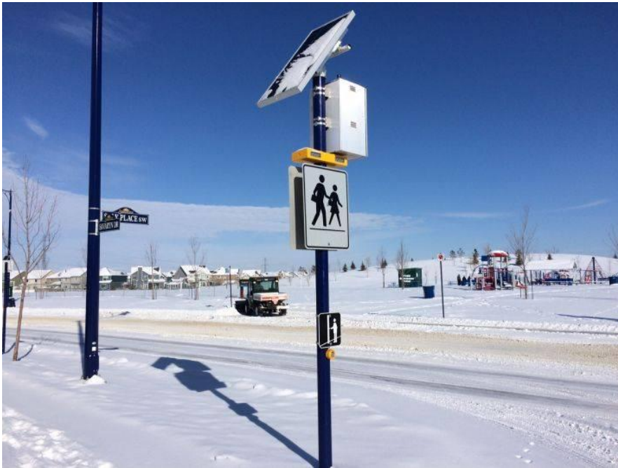
Figure 6: Rapid Flashing Beacons
