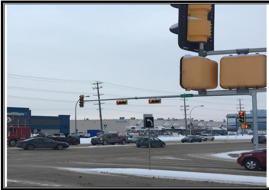
Figure 4: Full Traffic Signal
