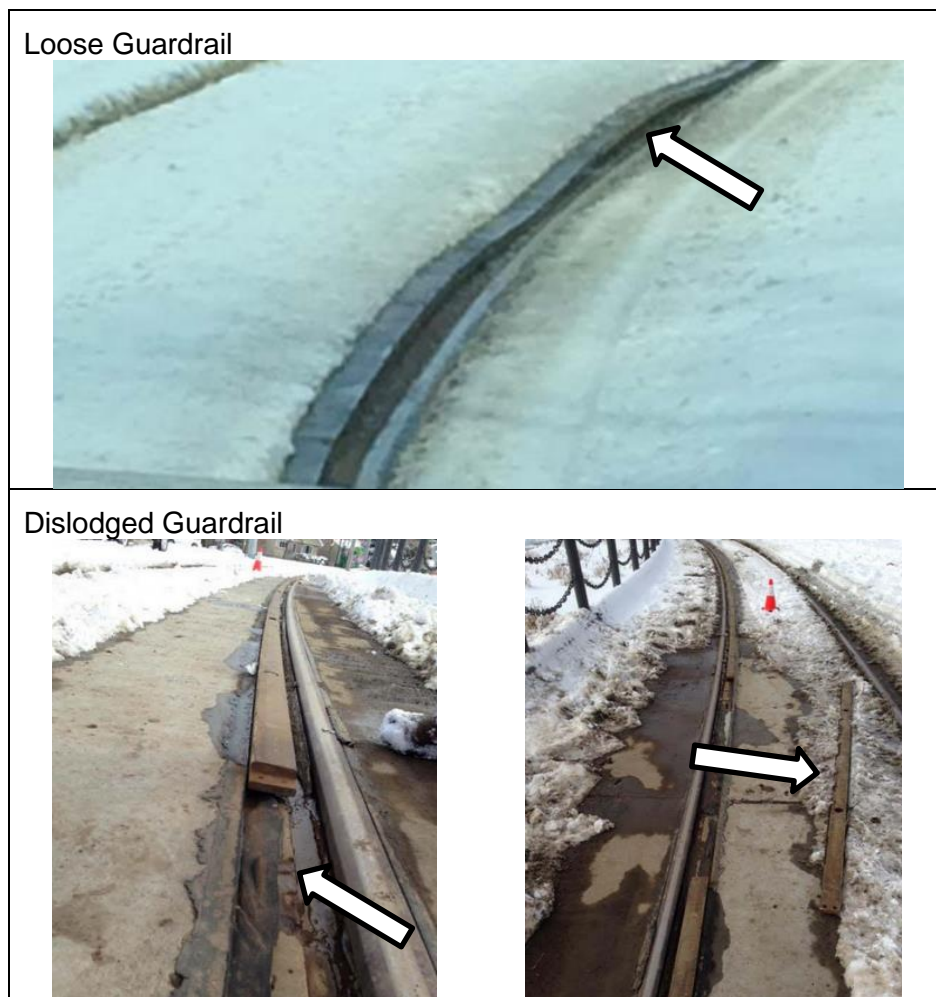
Figure 3 – Guardrail Track Issues
