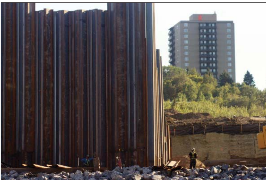
Workers standing next to sheet pilings on the south side demonstrate the scale of work involved in bridge construction.
