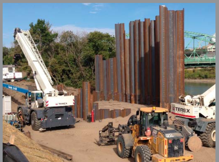
A square cofferdam takes form as sheet pilings are installed on the south side. Once all pilings are in place, soil inside is removed to create a dry work area.
