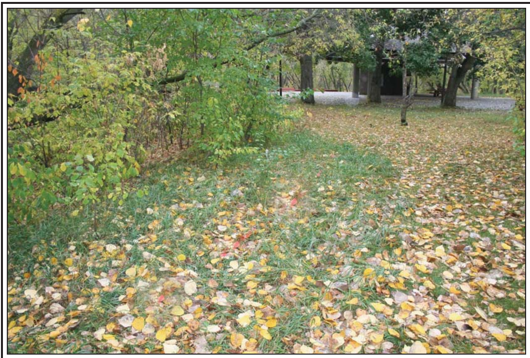
Photograph 7. View to the west showing the park building that the water line and electrical lines run towards from the emergency post and the water fountain. The intermittent orange line on the grass marks the buried pipeline identified by Alberta One-Call.
