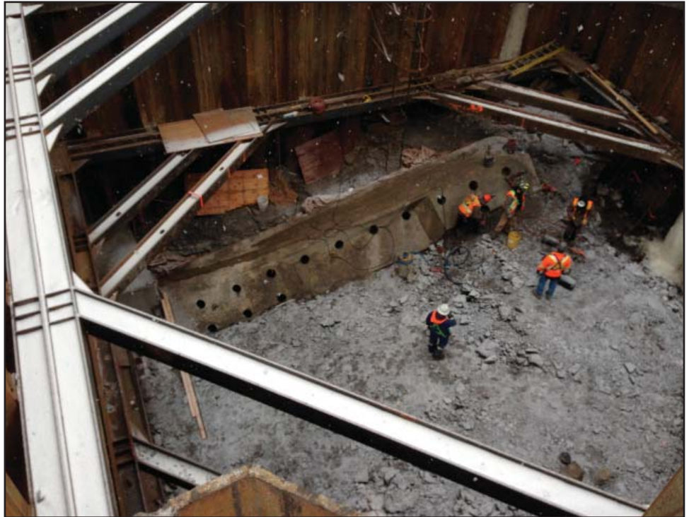
Northwest thrust block
