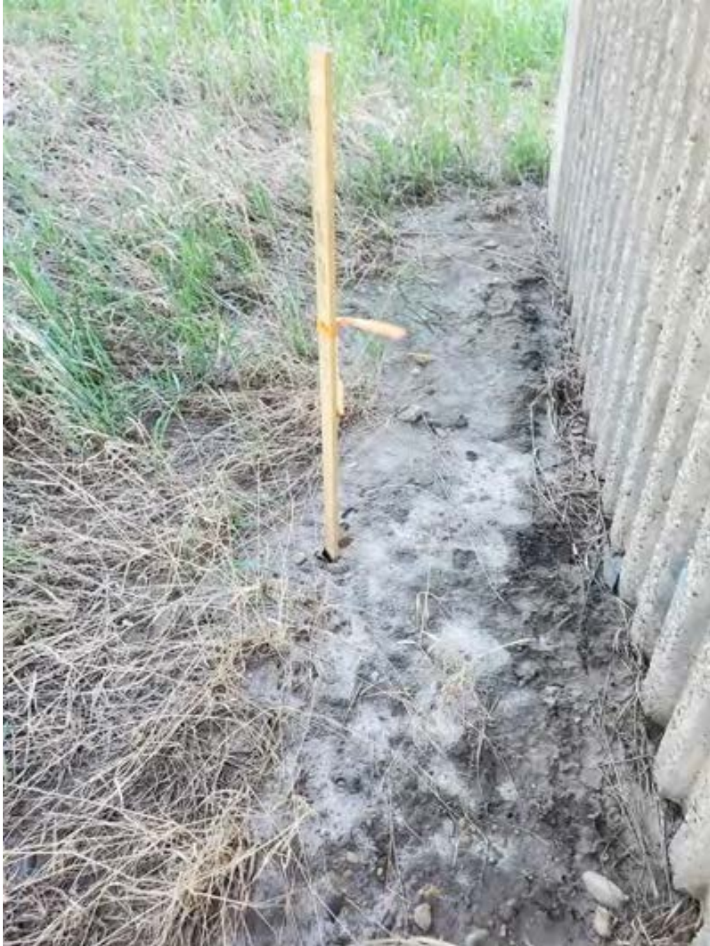
Photograph 3 – Salt staining at 21HA19, adjacent to pier below Rainbow Valley Bridges. June 4, 2021.
