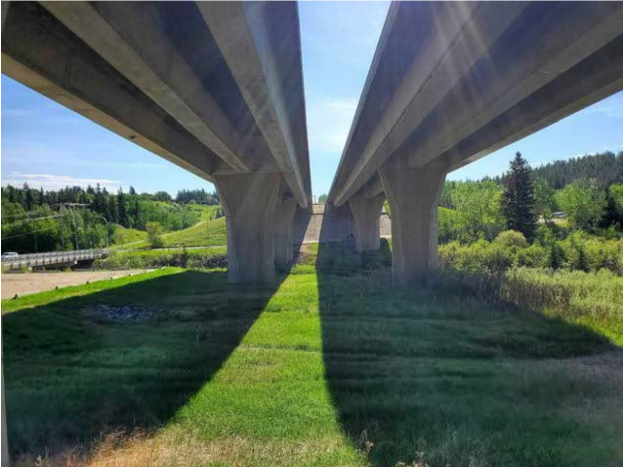
Photograph 2 – Rainbow Valley Bridges, facing east towards former spill area and 21HA13, 21HA14, and 21HA15 locations. June 4, 2021.
