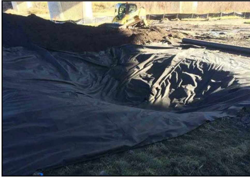
Photograph 7: A seepage pit was re-constructed with a non-woven geotextile liner beneath the drainage culvert on the Whitemud Drive overpass (October 21, 2016).
