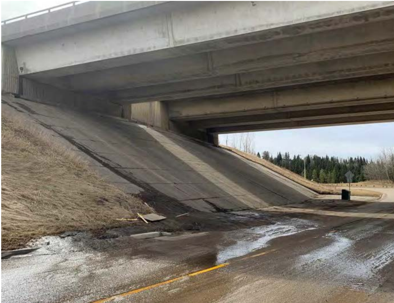
Photograph 7 – Facing southeast toward RVB, catch basin, box containing gravel, and cracks in lower concrete. April 22, 2020.
