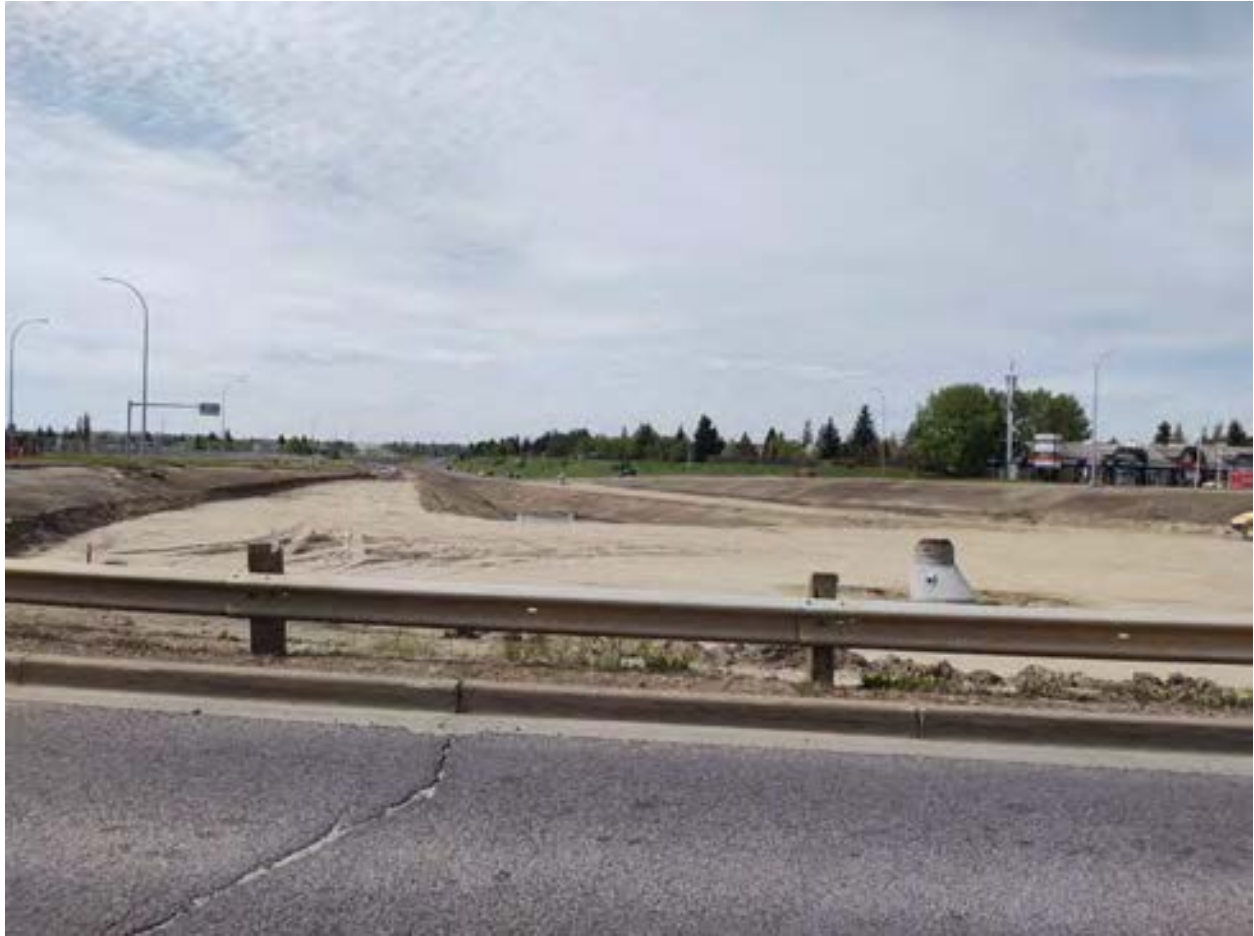
Figure 7. Construction area along Terwillegar Road, south of the project footprint, where vegetation cover had been removed. No obvious bedding could be observed, and the sediments appeared to be reworked.
