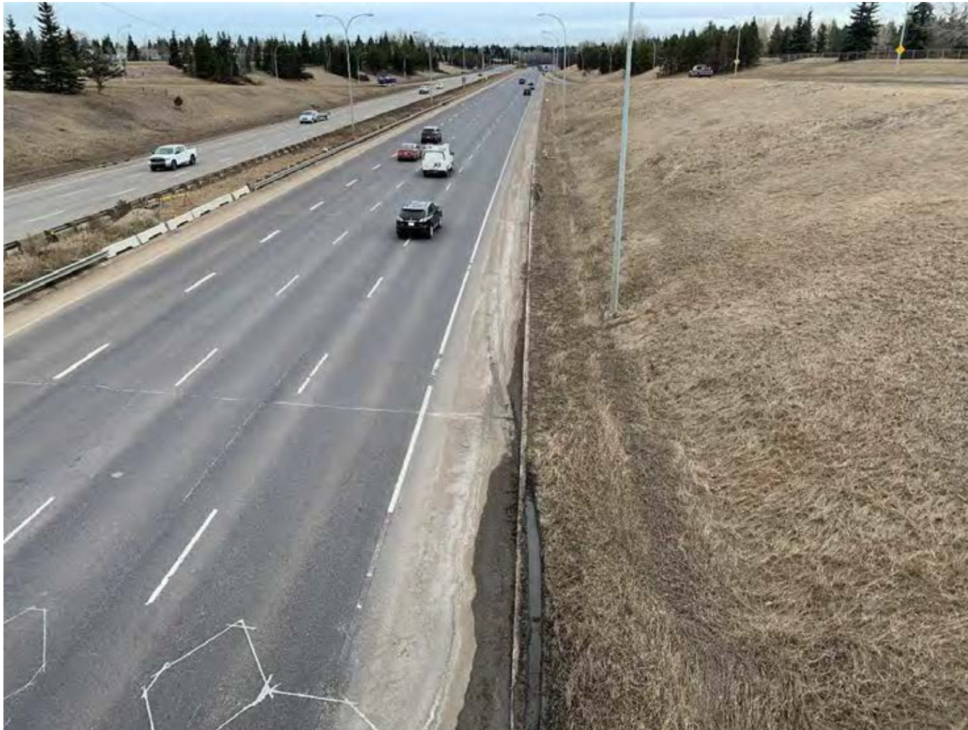
Photograph 3 – Facing north from 53 Avenue bridge, salt staining on WMD. April 22, 2020.
