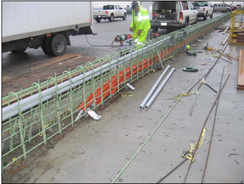
Figure 5 - Example of Conduit on Bridge Structure
