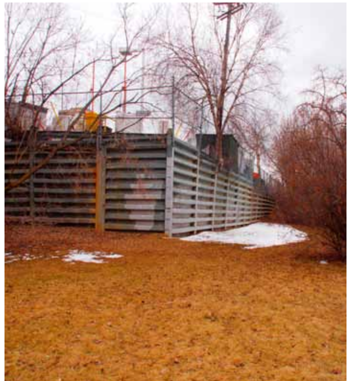
FIGURE 2.26: CONSTRAINT 6 - RETAINING WALL AT O'KEEFE SITE CREATES A DEAD SPACE IN THE ADJACENT PARK AREA.
