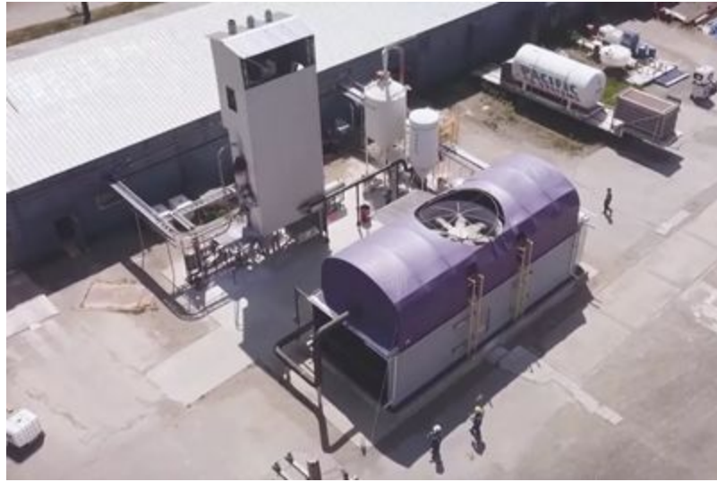
Carbon Engineering's pilot plant demonstrating Direct Air Capture of CO 2 in Squamish, BC 12
