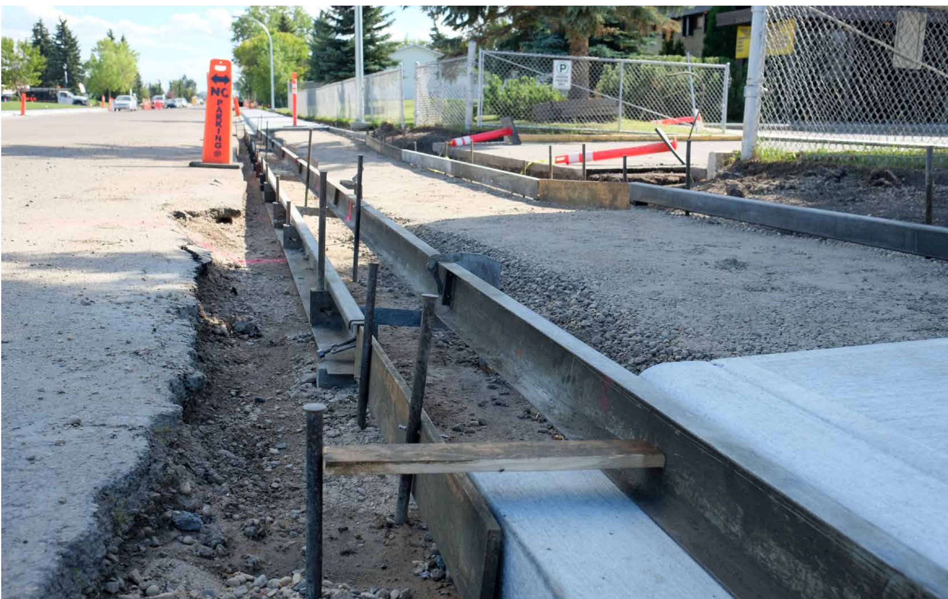
Forms are set in order to pour new concrete for the sidewalk.
