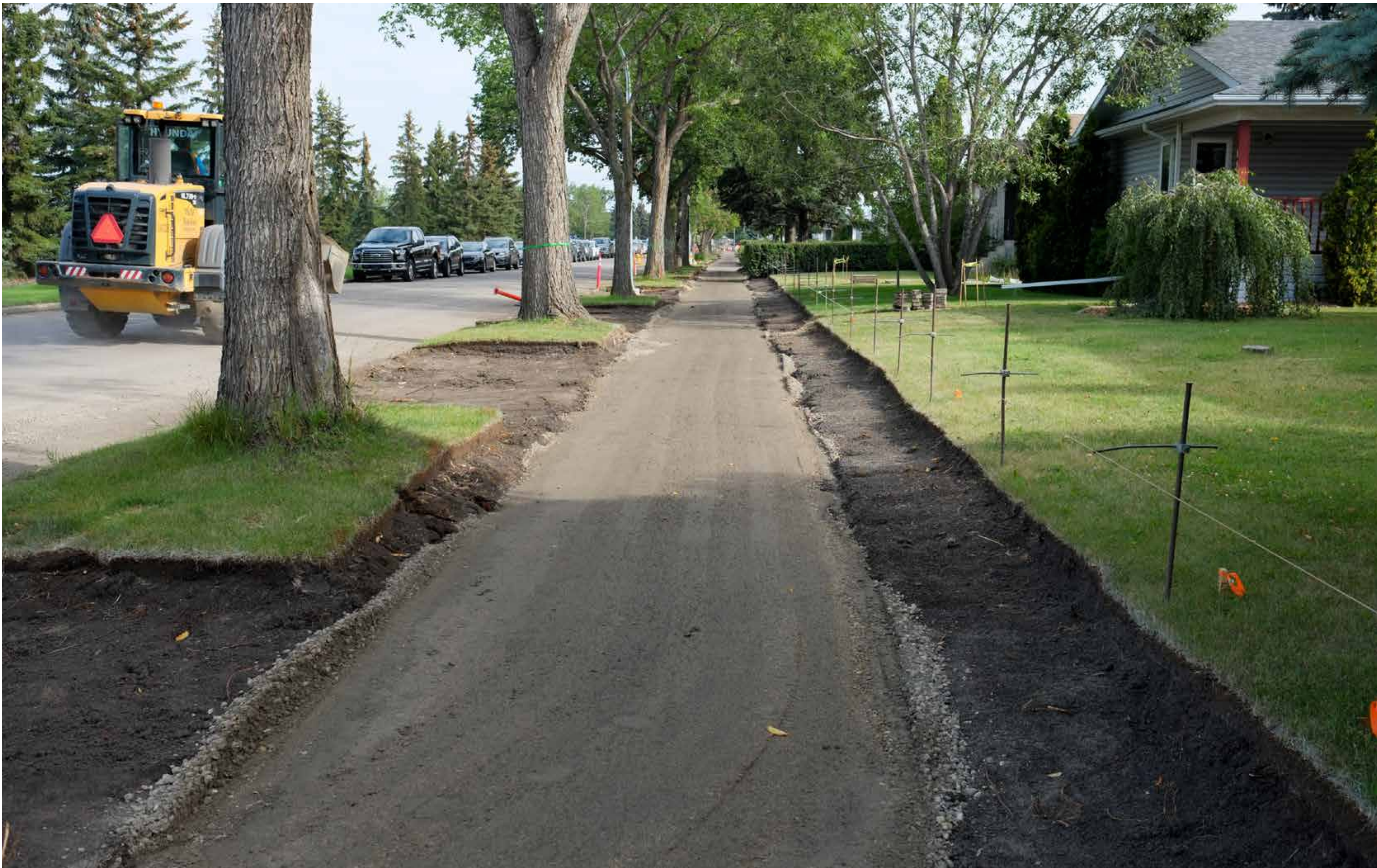
After removal of the existing sidewalk, gravel is placed and compacted to prepare for construction.
