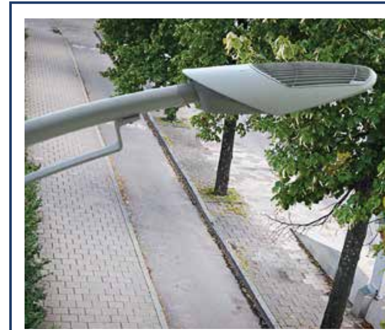
Roadway and Pedestrian Lighting Streetlight fixtures will be the same as those used on Jasper Avenue New Vision. Simpler poles will be used for both roadway and sidewalk lighting.
