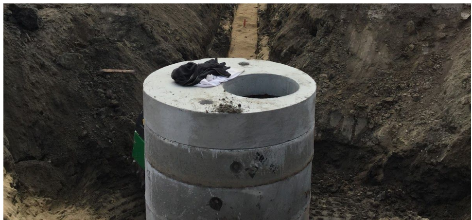
An example of utilities excavation that may be required for this project.
