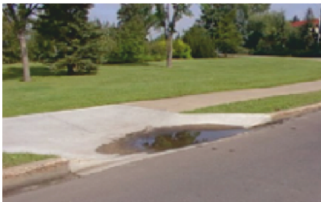
Standing water in crossing is unacceptable
