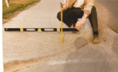
Curb ramp > 6.0% crossfall
