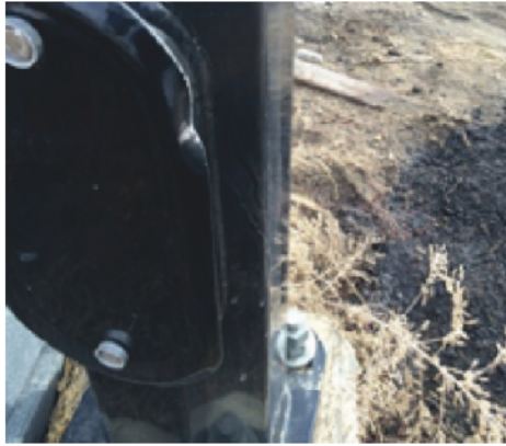
Damaged hand hole cover
