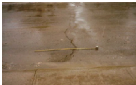
Open asphalt joints causing riding quality
