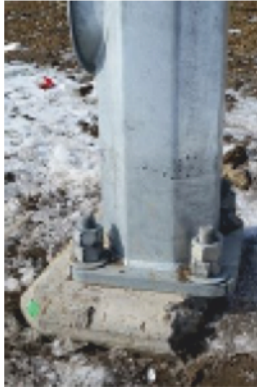
Damaged precast base
