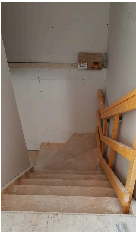
This stairway has a continuous, graspable handrail for its full length. With the opposite side being a closed wall, this is safe.
