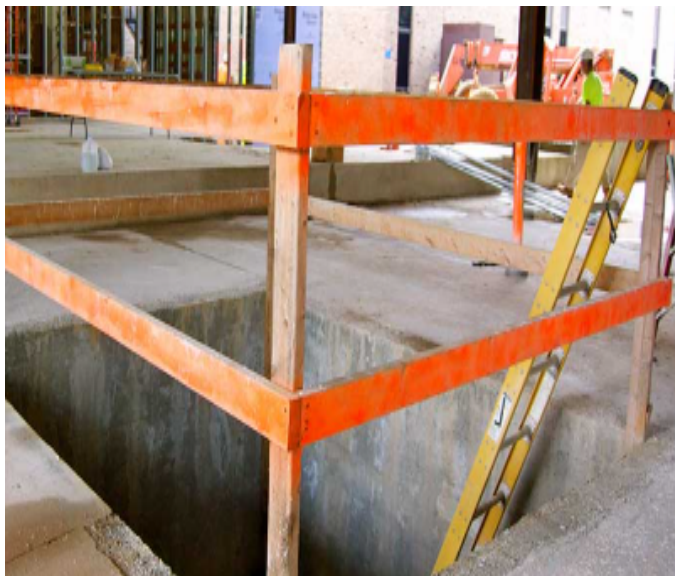
Example of proper opening protection with guardrails.
