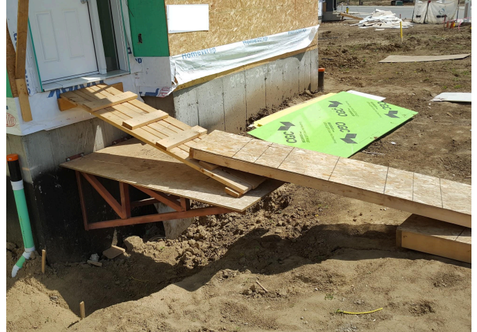
Lack of handrail and an open excavation make this unsafe.
