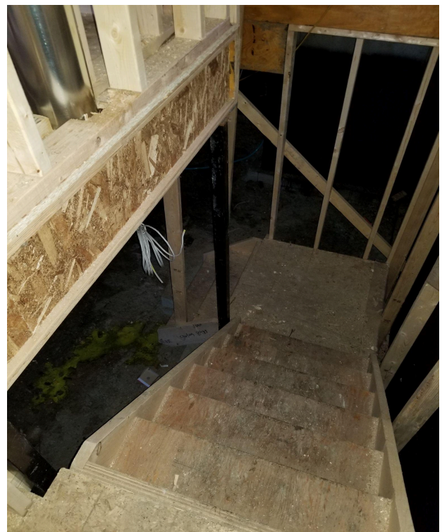
This stairway has 5+ risers, making a handrail mandatory. Note: Open framing/studs on the side do not constitute a handrail. A secured, graspable rail must be installed at 800mm–920mm height (2.62-3 ft).
