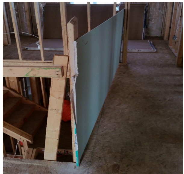
No solid guardrail or rigid material to prevent a fall.
