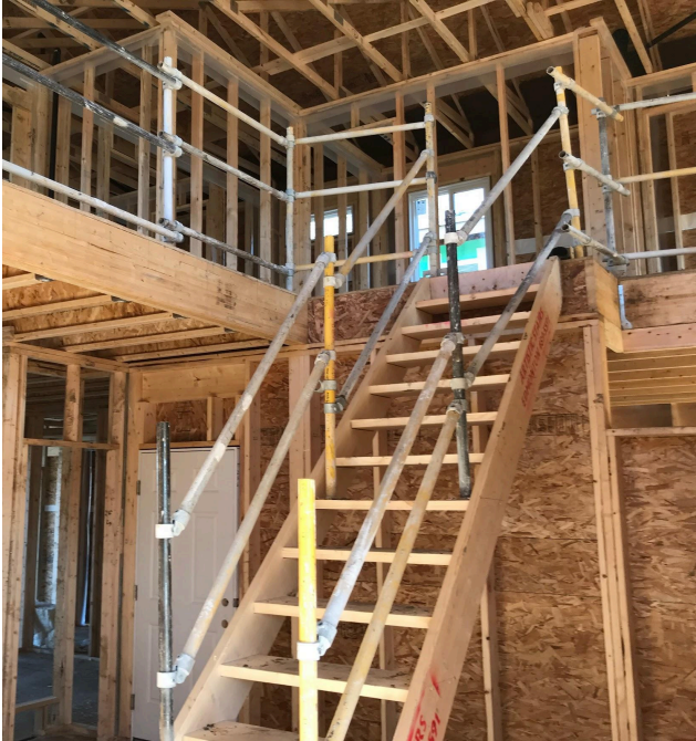
Handrails on both sides, firmly anchored for safe access.
