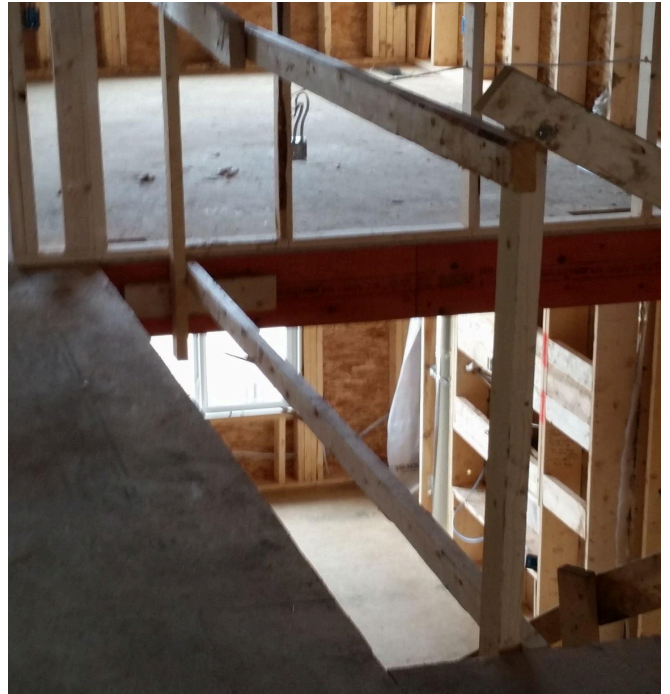
Guardrail is not to the edge of the opening leaving a fall hazard.
