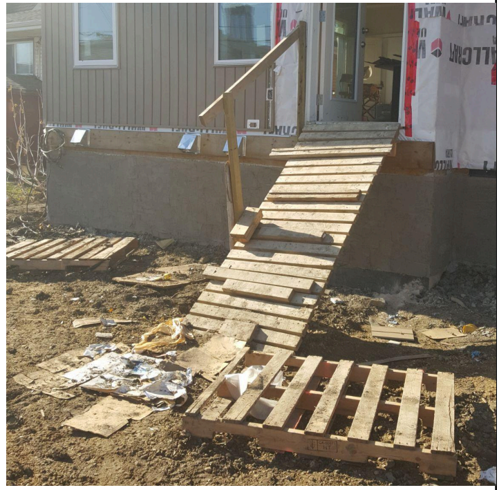
Non-continuous and missing handrail make this unsafe.
