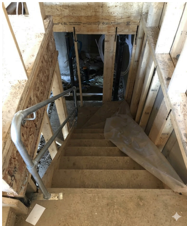
This stairway has 5+ risers, making this a handrail mandatory. Note: Open framing/studs on the side do not constitute a handrail. A secured, graspable rail must be installed at 800mm–920mm height (2.62-3 ft).
