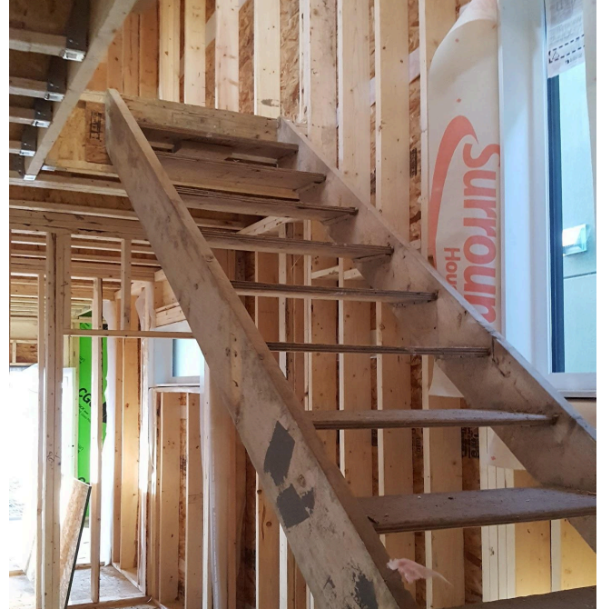
This stairway has 5+ risers, making a handrail mandatory. Since both sides of this stairway are currently open, a handrail is needed on both sides (unless one side is walled in).
