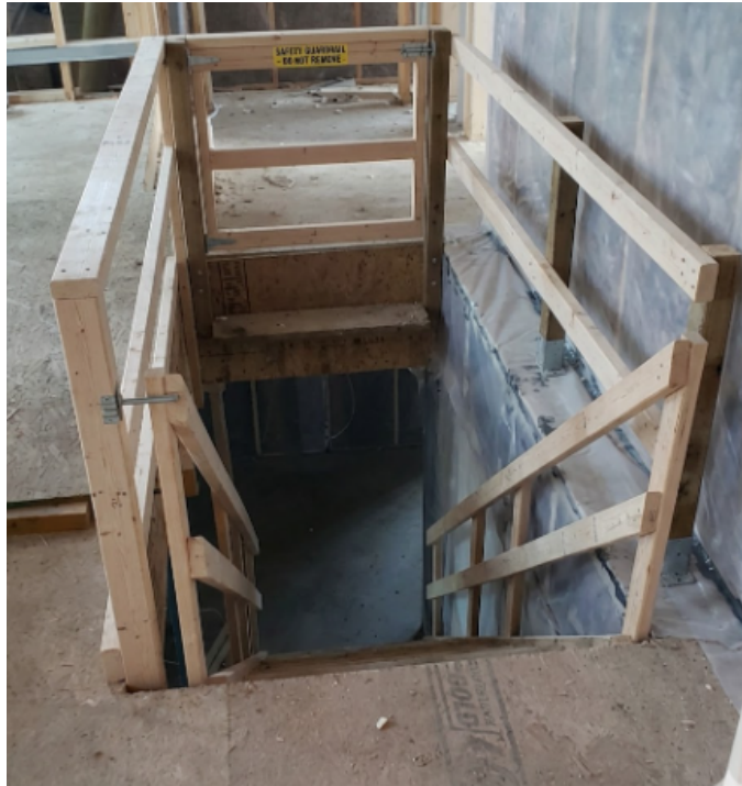
Guardrails are in place around the floor opening and going down the stairs.
