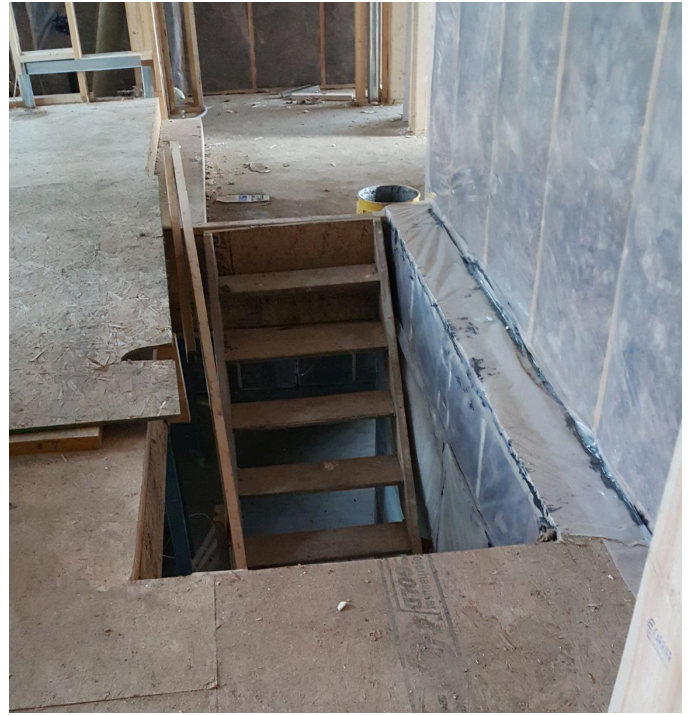
No guardrails around the floor opening and no handrail on stairs.
