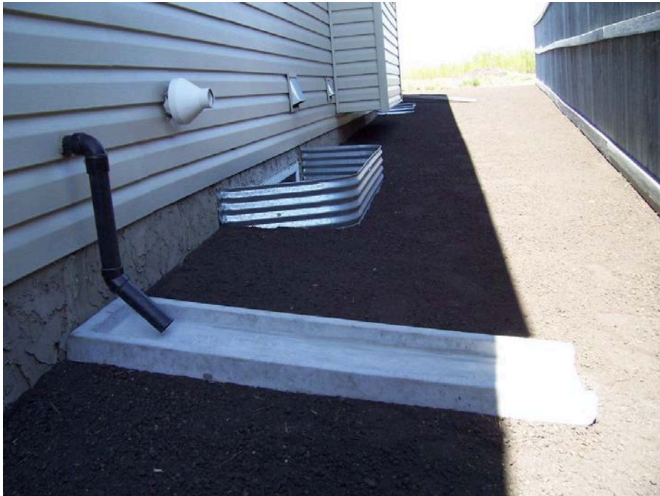
Figure 19 - Splash pad under sump discharge
