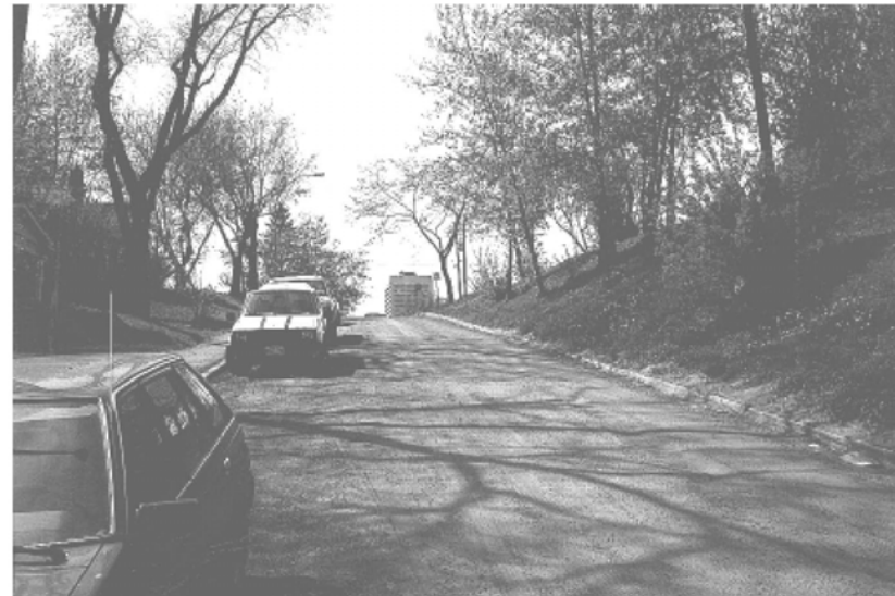
100A Avenue is in need of repair
