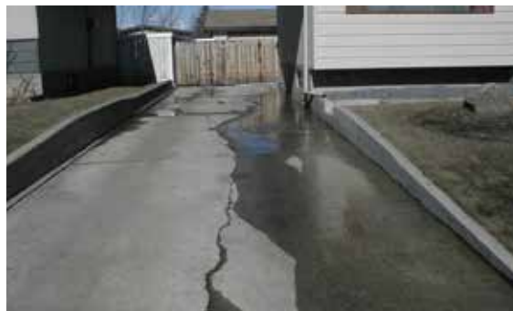
Property on right with negative grade and evidence of surface runoff at foundation wall
