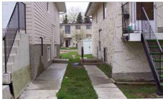
The sump pump discharge on the left drains towards the right property, which has a slope towards the foundation wall.
