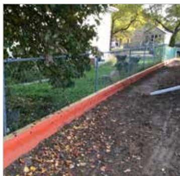
Example of internal swale and retaining wall at rough grade with moisture barrier
