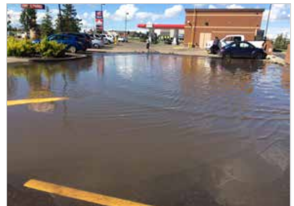
Stormwater is stored and drains slowly into a catch basin during and after storm events.
