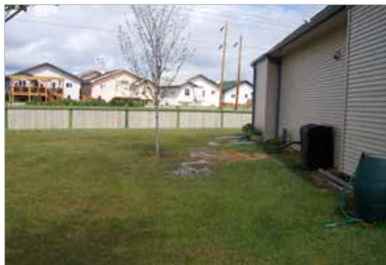
Settlement beside this condominium unit causes water pooling and potential basement flooding
