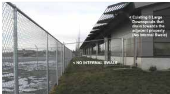
This new commercial development with surface drainage flowing towards the adjacent property is in violation of the Bylaw.
