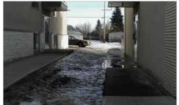
Poor lot grading between two apartments creates a low area for ponding during snow melt
