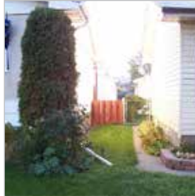
This downspout directs storm-water towards a neighbour's lot, which has a slope towards the foundation wall.
