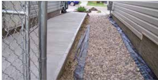
This new sidewalk does not have 15 cm drainage space within the property.
