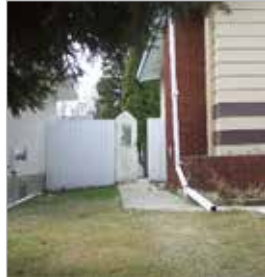
With a slope towards the foundation on the left, stormwater will flow towards the left house.
