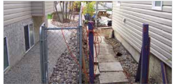
The new sidewalk on the left has the minimum 15 cm drainage space requirement within the property that drains surface runoff towards the street.
