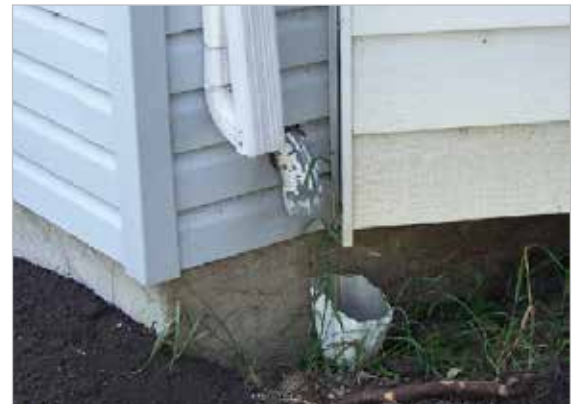
Downspout disconnected from storm service
