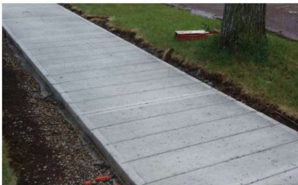
▲ Extra deep cuts and rebar are added to the sidewalk to control where the sidewalk will crack and to keep the sidewalk intact as the tree's roots grow.
