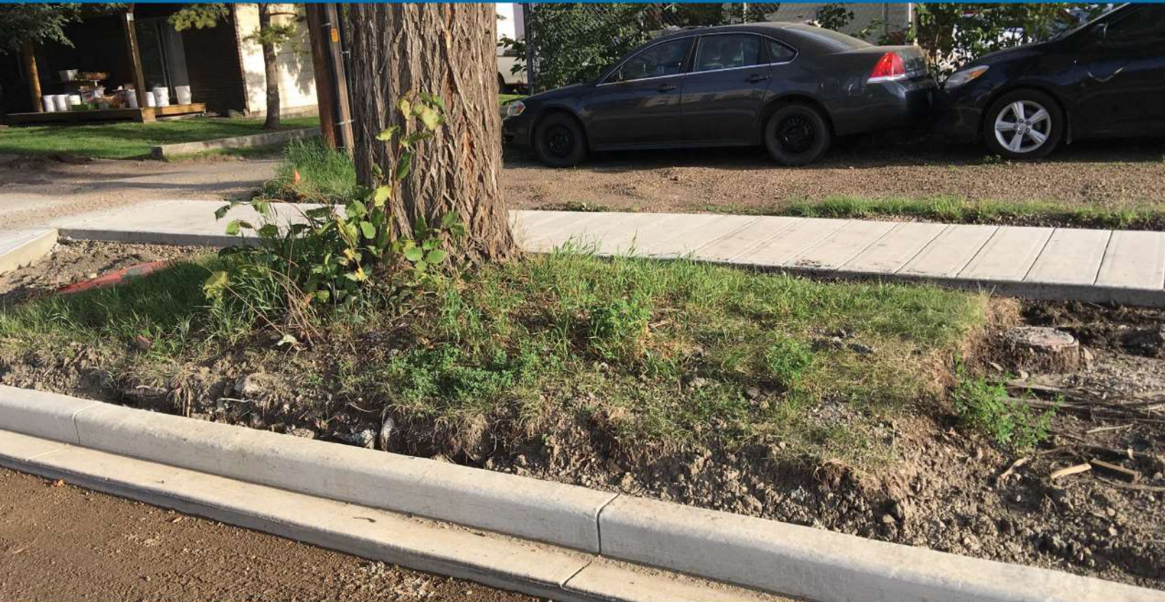
▲ An area around each tree is maintained during construction to protect it and its roots.
