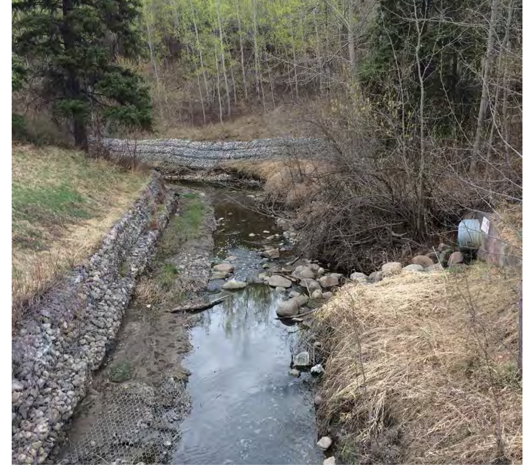
Undermining of erosion protection
