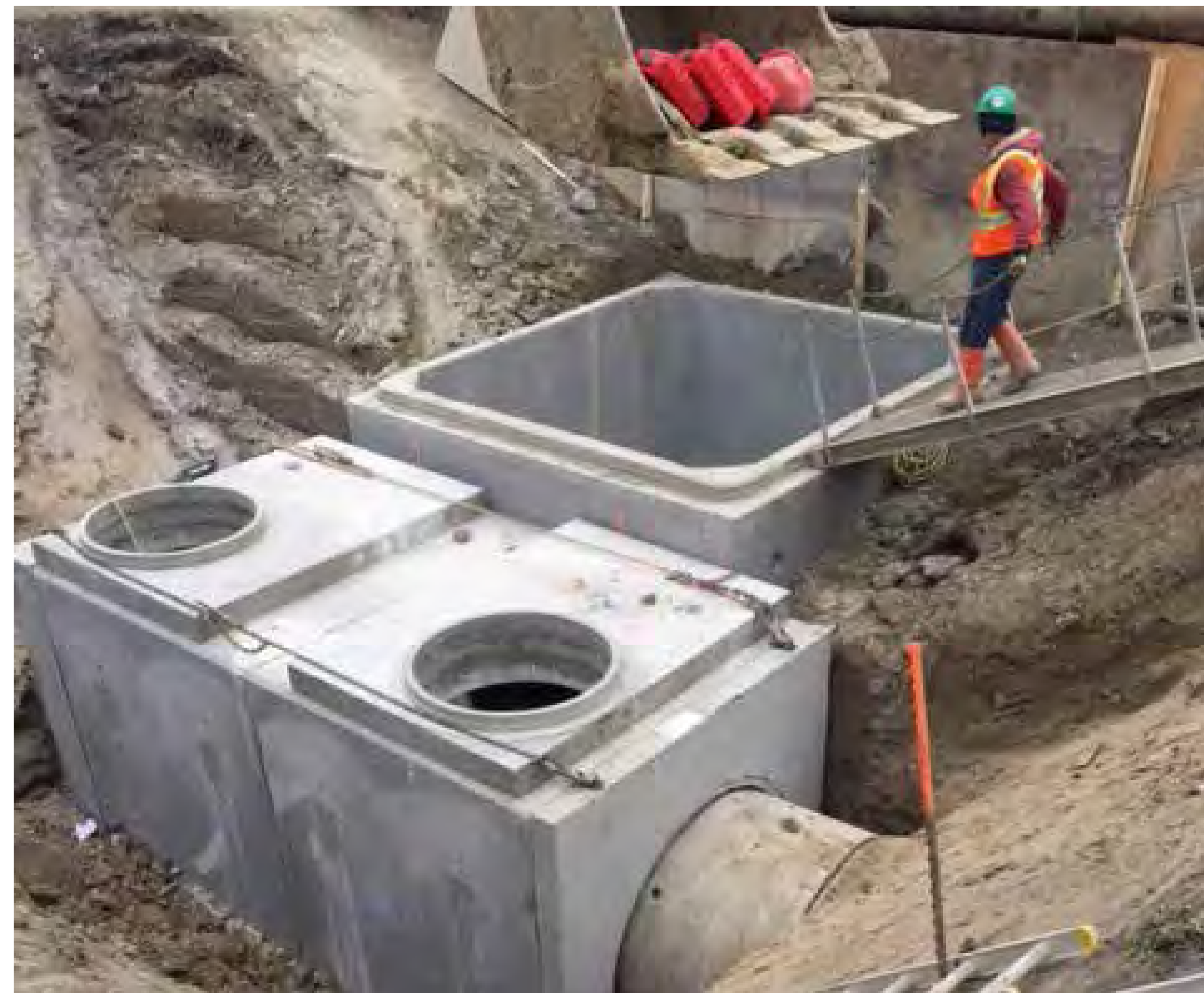
Underground oil and grit separator
