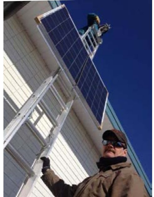
Warren Saurer, chair of the Solar Society of Alberta, helps with the installation at Meadowlark hall
