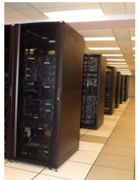
City of Edmonton's main data center is 7,500 square feet and is home to servers that safely store the City's information.
