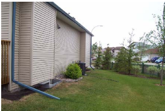
Roof drainage violation from a condominium property onto a City right-of-way. Roof drainage must drain on-site towards catch basins.
