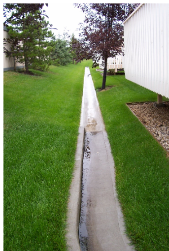
A concrete drainage swale at the back of condominium units on a multi-family site
