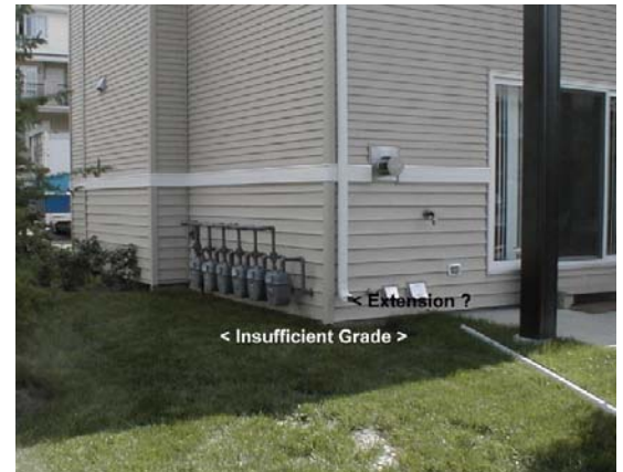
Insufficient grade away from a multi-family project
