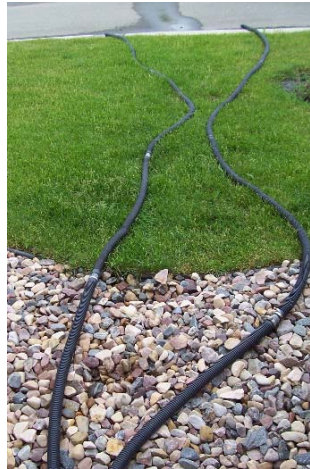
Sump Pump discharge hoses at a multi-family site with discharge to common private road
