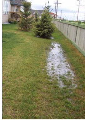
Pooling on an internal swale at a commercial property
