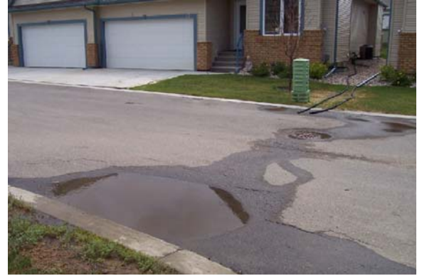
Settlement on private roadway near and around the catch basin at a multi-family property
