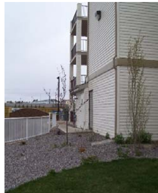
Roof drainage of an apartment violation. Roof drainage must not Drain towards City or adjacent lots.
