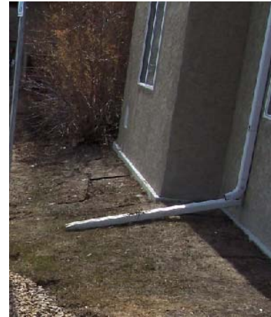
Downspout with an extension at an apartment
