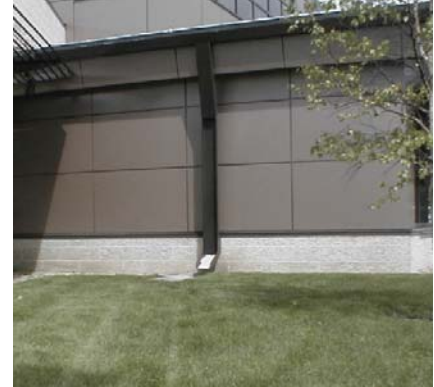
Downspout at a commercial building
