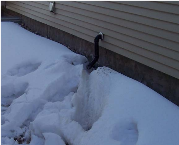
Sump Pump discharge at a condominium in winter
