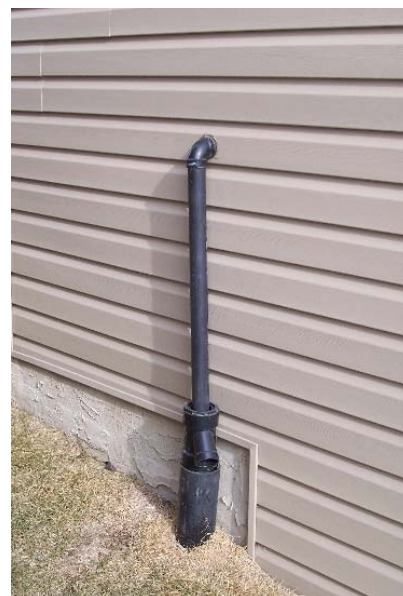
Sump Pump to storm service multi-family site
