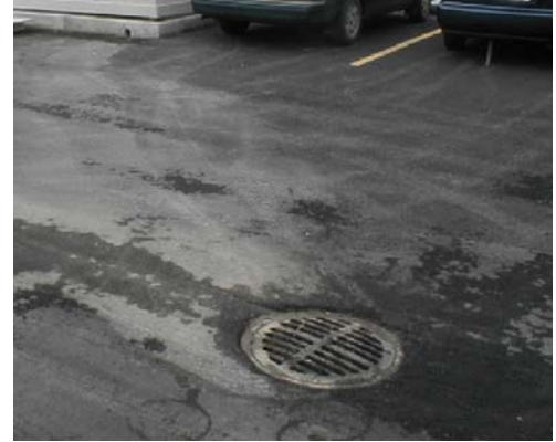
Apartment parking lot with a catch basin
