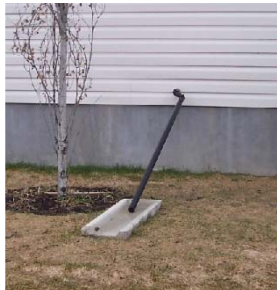
Sump Pump discharge at a condominium site
