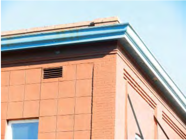
>> South west cornice
